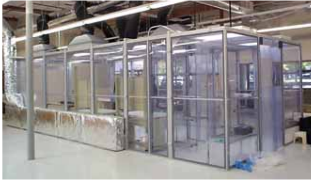
Rather than ceiling plenums and air chases in the walls, this room uses an elaborate system of ducting to recirculate air leaving the room, and bringing it back in through the ceiling to pass through the HEPA filters before re-entering the room. The gowning area on the right end of the room provides technicians a place to gown before entering the main cleanroom, reducing the risk of contamination.
