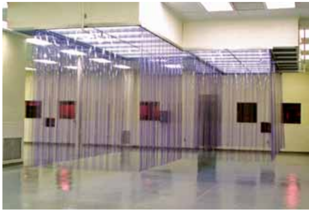
This enclosure is in As Built state, before equipment and materials are moved in. Notice that it is within an existing room and takes advantage of the air conditioning infrastructure that is already installed. Cleanrooms are certified by the manufacturer in an As Built state.
